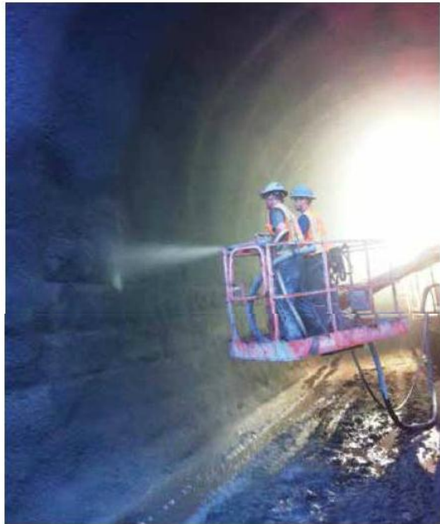
Fig. 3: Manlifts used to access the arch roof for scaling, drainage placement, and shotcreting
